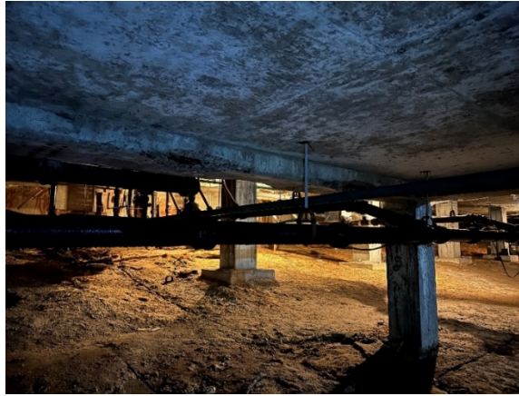
Figure 2 Concrete Beam Spalling Damage
