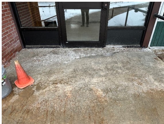
Figure 6 South Entrance Concrete Damage
