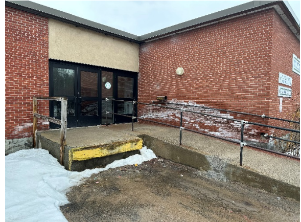
Figure 8 East Entrance (1993 Addition) Concrete Damage
