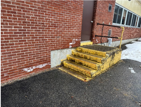
Figure 7 North Entrance Concrete Damage
