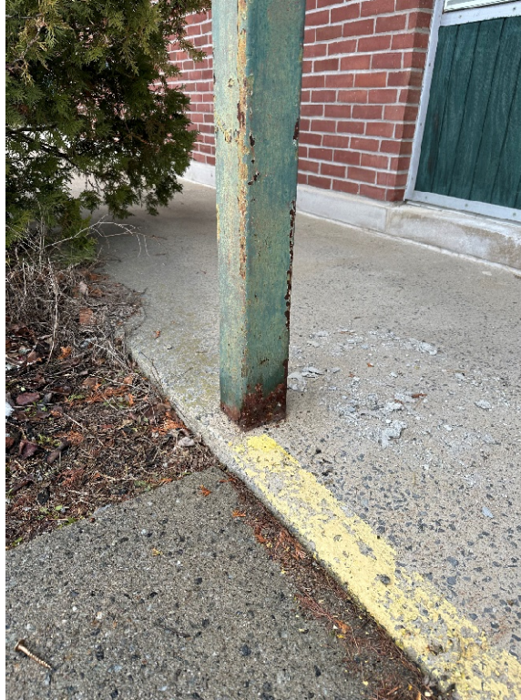
Figure 5 Steel Column Corrosion
