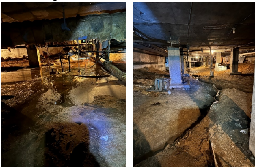
Figure 3 & Figure 4 Water Infiltration in Crawl Space
